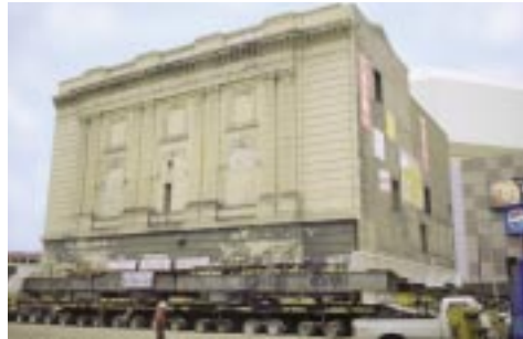
The Shubert Theater in Minneapolis, Minnesota, was positioned onto its new foundation with the assistance of 70 dollies and 100 hydraulic jacks equipped with Aeroquip jack hose. (Photo by Artspace Projects, Inc., Minneapolis, MN, © copyright 1999)
